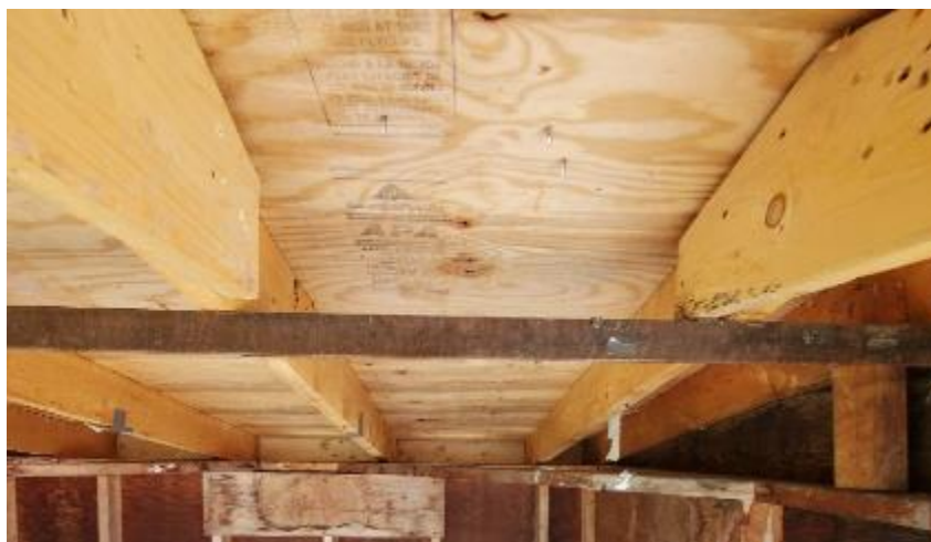
Photo No. 12 Post Test Underside
