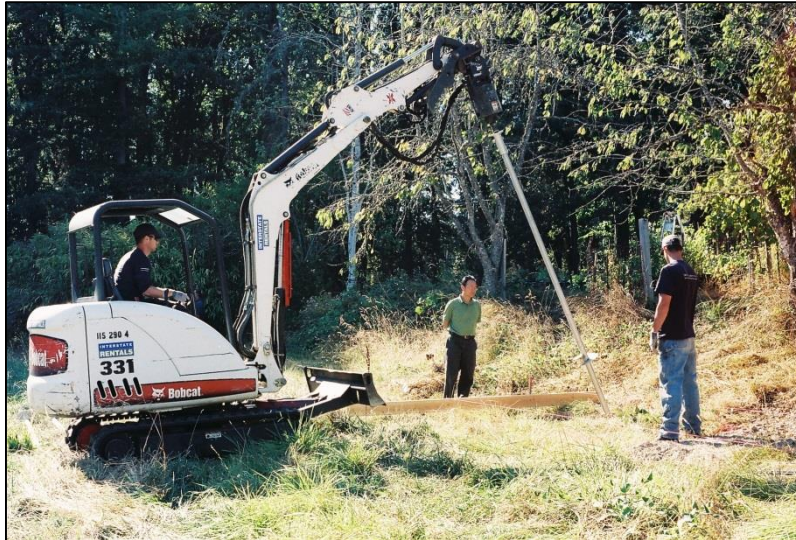
Figure 4 – A small Bobcat 331 being used to drive a 10 ft auger using the technique of advancing upon the auger to vertical as it is driven.
